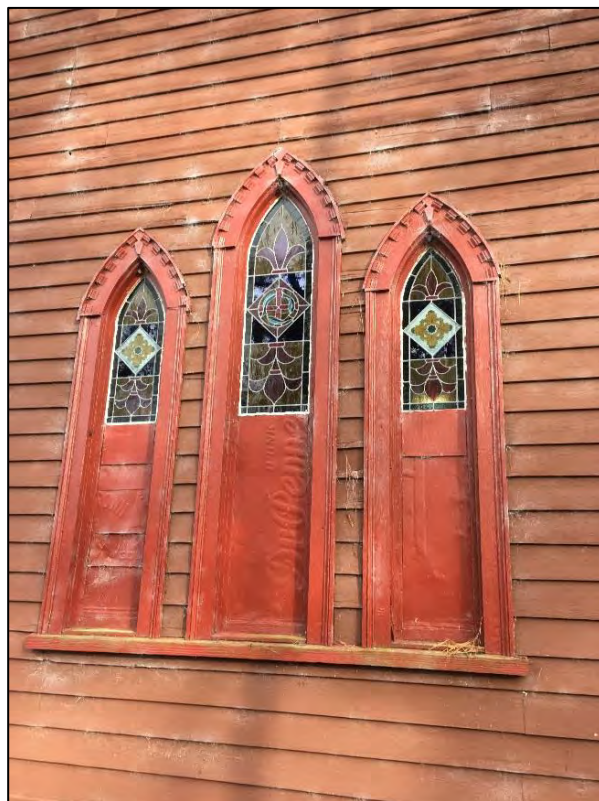
Figure 40. Detail view of west elevation window, St. John's Episcopal Church, facing east.
